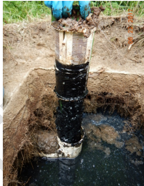
Illustration 2 – Clogged Effluent filter
