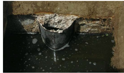
Illustration 1 - Concrete Corrosion Around Outlet Baffle
