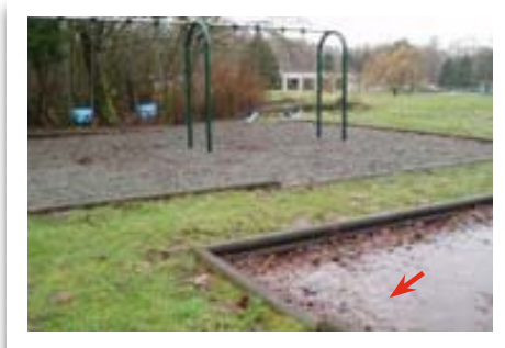
Poor drainage creates barrier and hazard. PHOTO COURTESY OF SHIRA STANDFIELD
