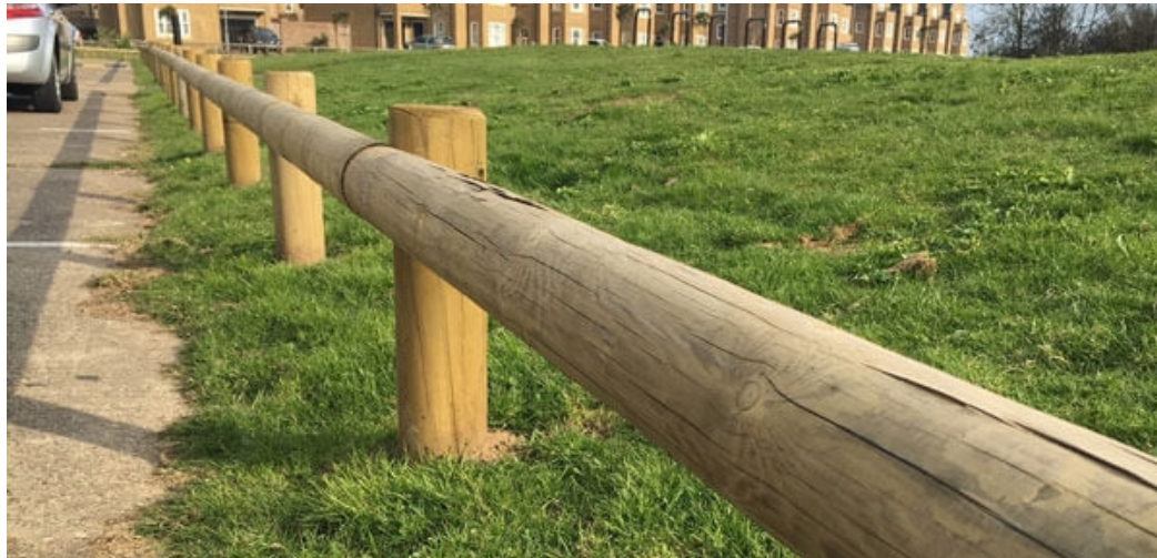
Figure 2: Example of standard treatment of edge protection (Final installation may appear differently than the figure above.)
