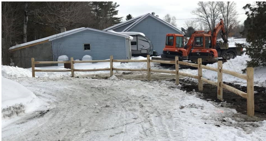
Figure 1: Post and rail edge protection on K&P Trail – Corner treatment
