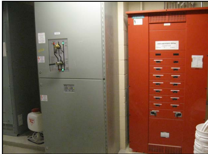
Photo No. 25: Emergency power 347/600V main distribution panel and automatic transfer switch
