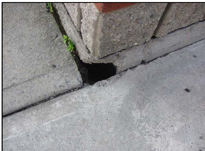
Photo No. 4: Deteriorated foundation wall
