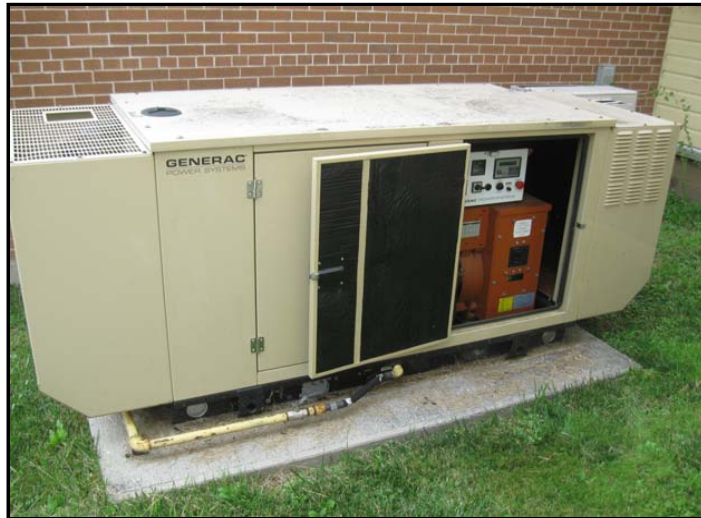
Photo No. 21: Generator
