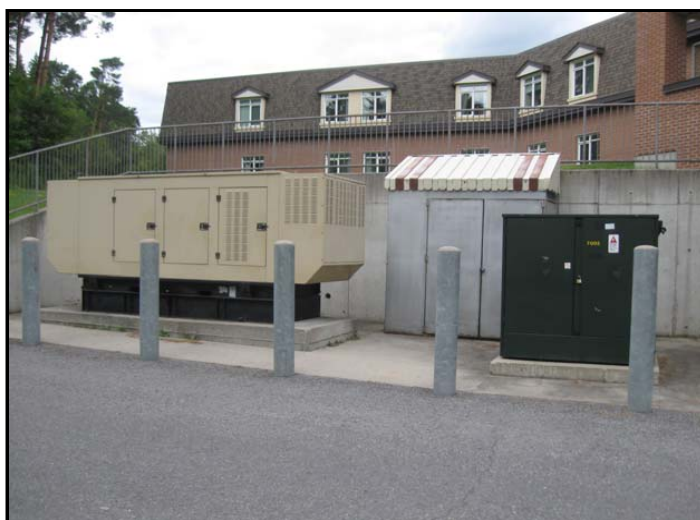
Photo No. 24: Generator and pad-mounted transformer
