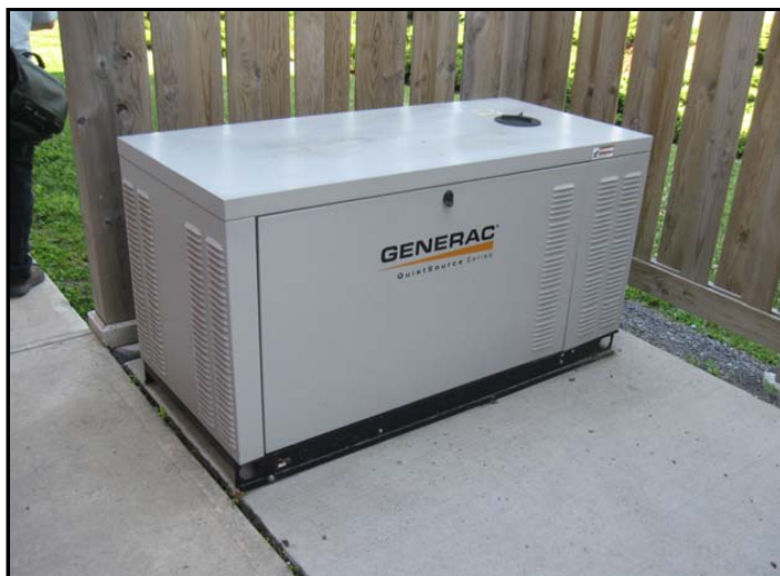
Photo No. 16: Generator
