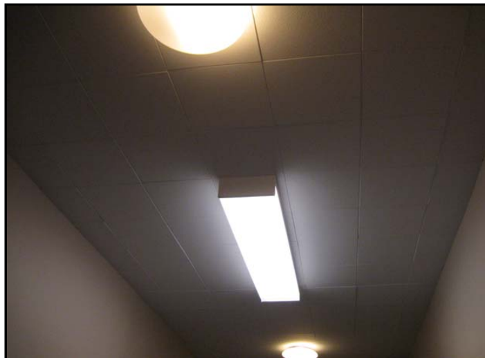
Photo No. 34: Second floor corridor lighting
