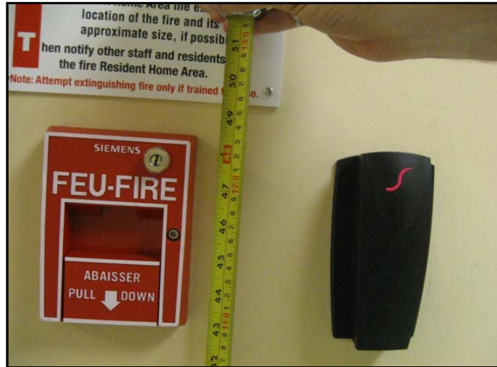
Photo No. 21: Fire alarm pull station
