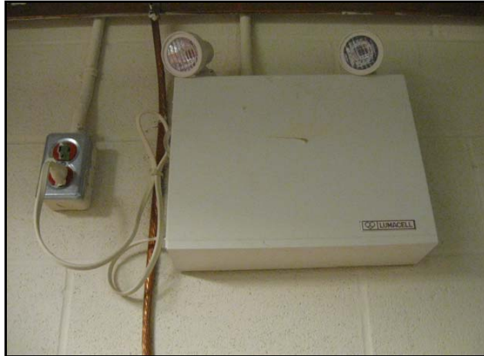
Photo No. 27: Emergency lighting wallpack
