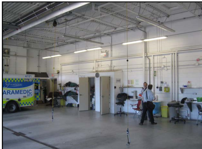
Photo No. 38: Garage lighting
