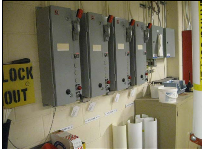
Photo No. 53: Motor starters
