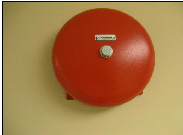
Photo No. 22: Typical fire alarm bell
