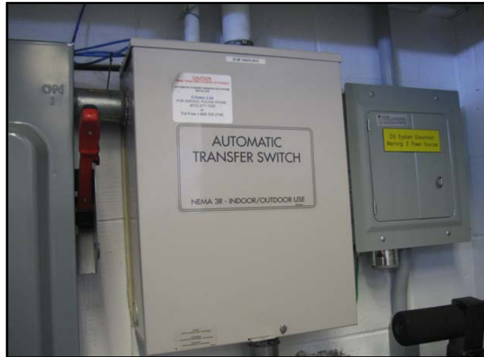
Photo No. 17: Automatic transfer switch
