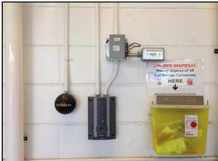
Photo No. 29: Garage gas detection system
