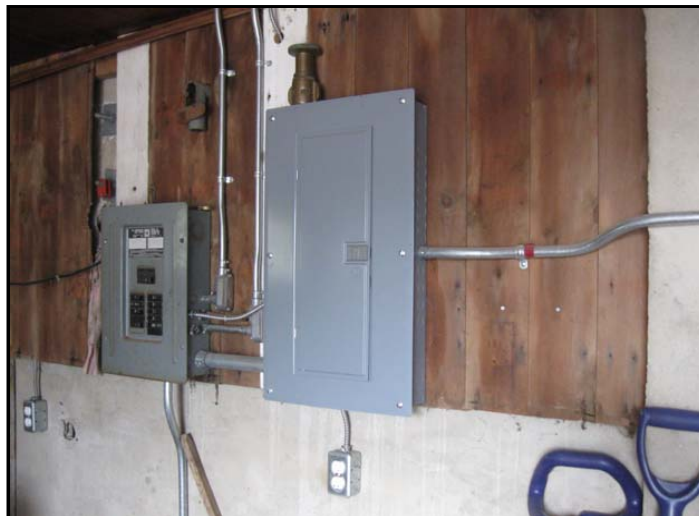
Photo No. 18: Garage electrical panels
