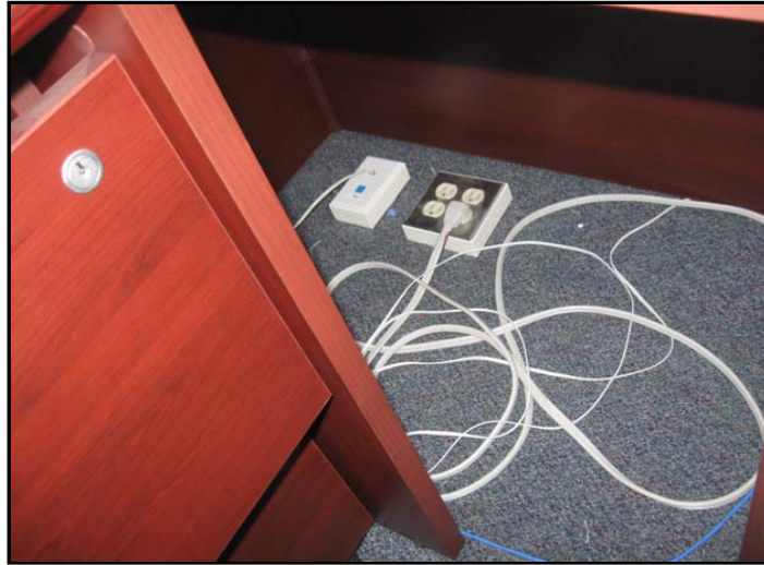
Photo No. 31: Office receptacles
