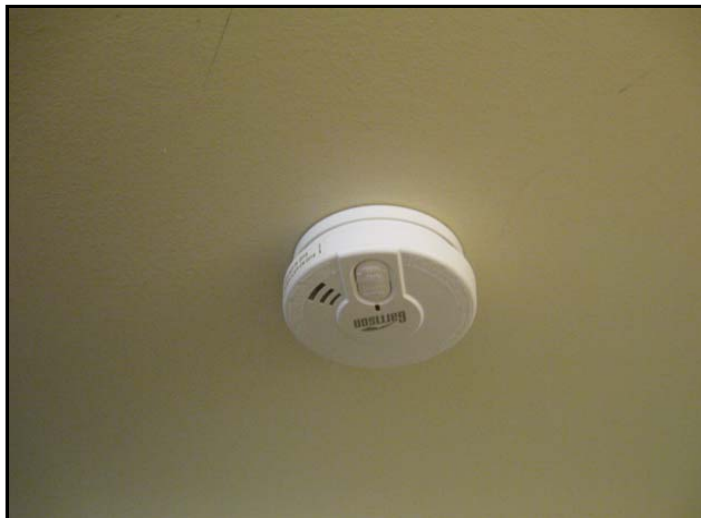
Photo No. 13: Smoke alarm
