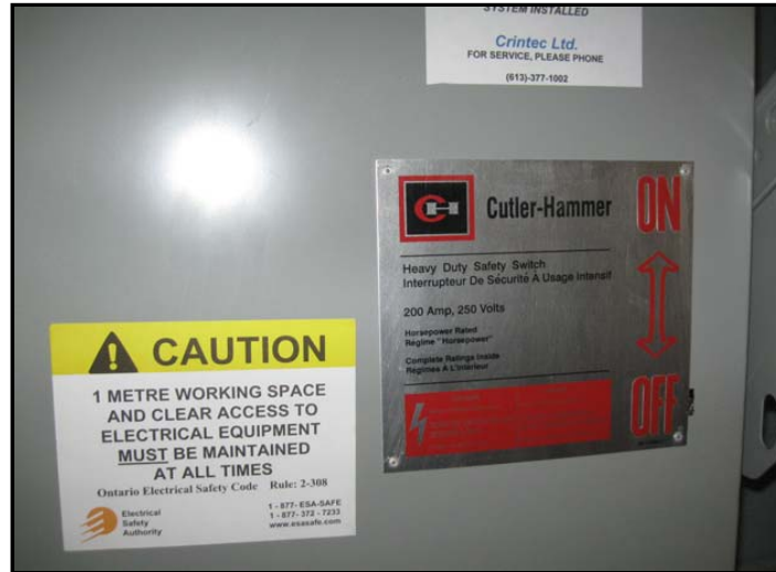
Photo No. 29: Main electrical switch
