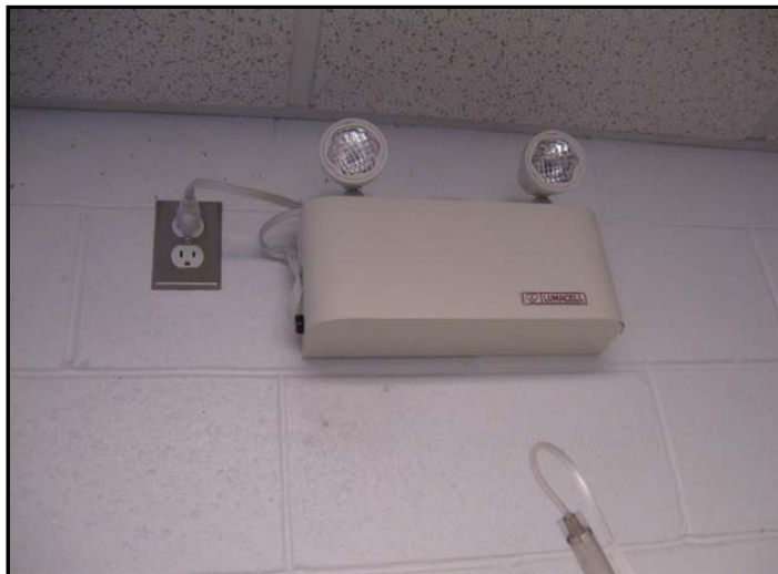
Photo No. 15: Emergency lighting wallpack
