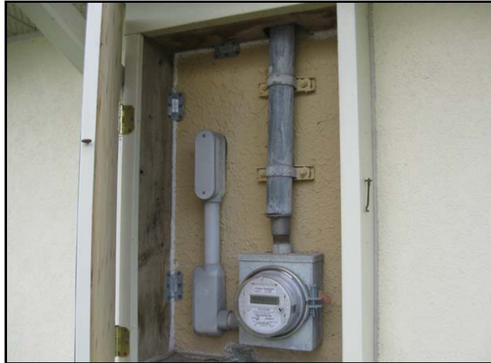
Photo No. 17: Garage electrical meter
