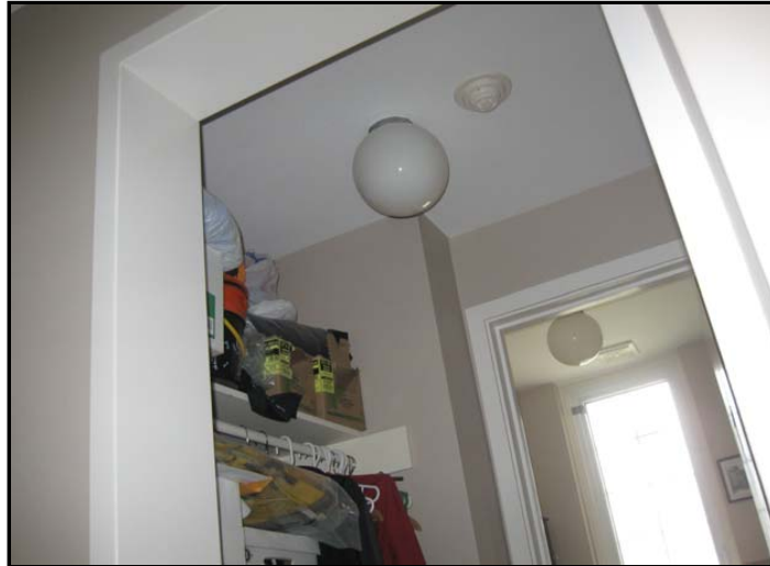
Photo No. 33: Ceiling-mounted decorative lighting
