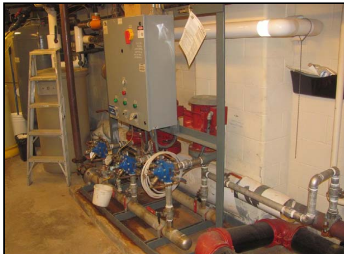
Photo No. 50: Domestic booster pump
