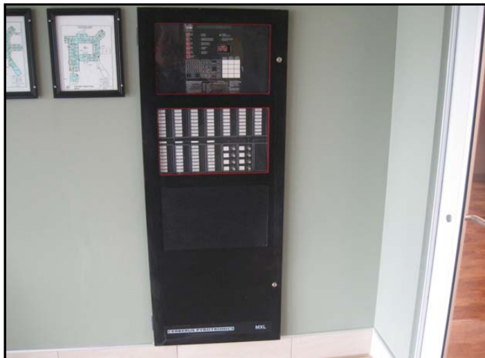
Photo No. 19: Fire alarm control panel
