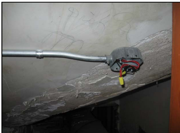
Photo No. 20: Attic heat detector or cover plate missing
