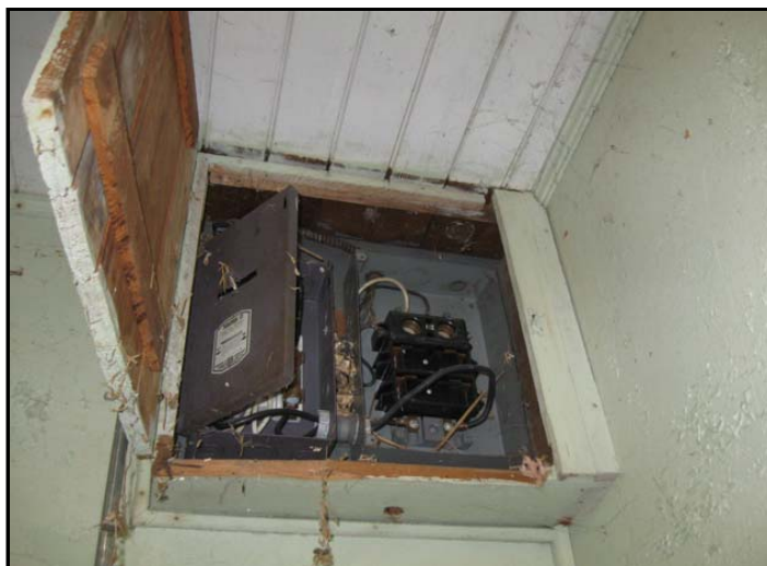
Photo No. 20: Abandoned panel in shed
