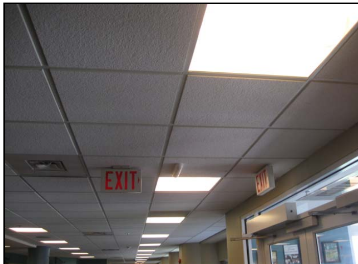
Photo No. 58: Ground level reception area lighting
