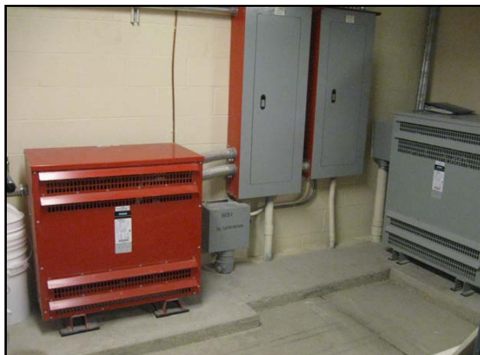
Photo No. 26: Emergency power transformer and panels
