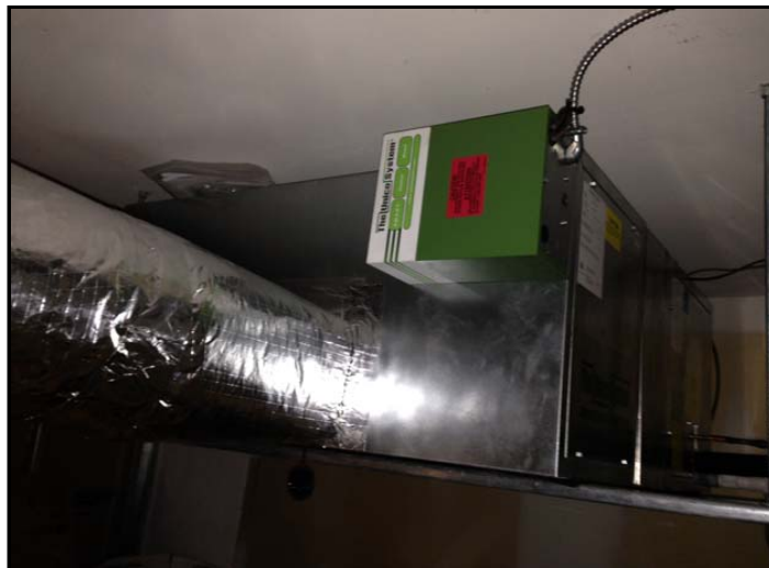
Photo No. 28: Ground floor fan coil unit
