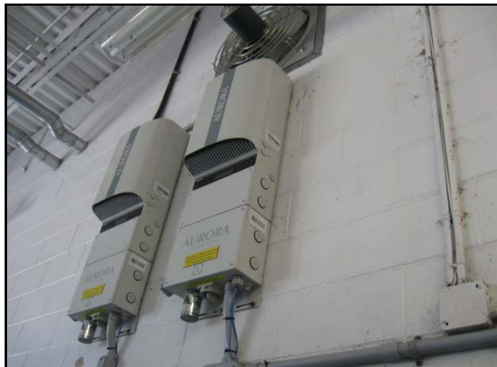
Photo No. 36: Photovoltaic equipment
