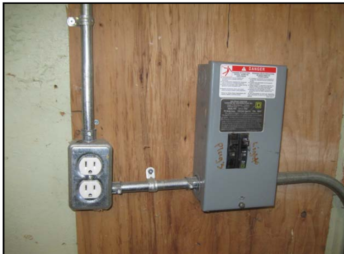
Photo No. 19: Shed electrical sub-panel
