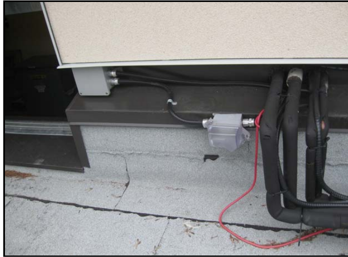
Photo No. 57: Rooftop receptacle at Auditorium
