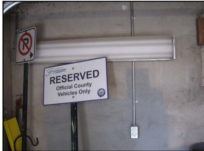
Photo No. 21: Garage interior wall-mounted lighting
