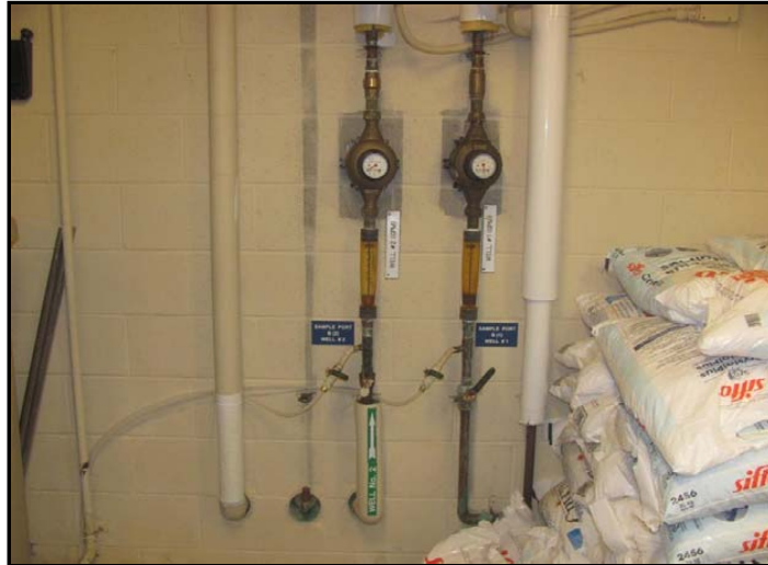
Photo No. 49: Incoming well water
