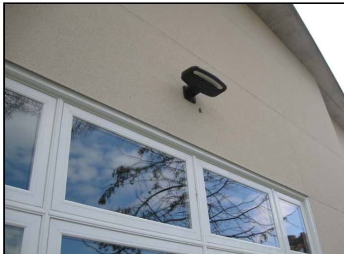
Photo No. 62: Exterior LED lighting at Auditorium
