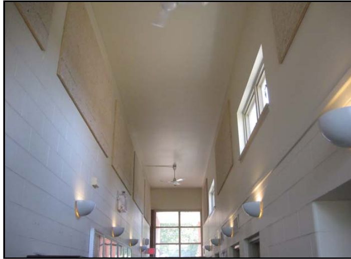
Photo No. 37: Corridor lighting
