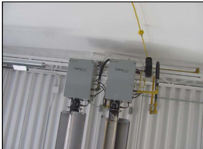
Photo No. 32: Gas-fired radiant heaters
