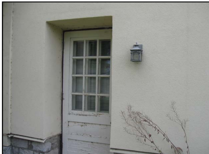
Photo No. 36: Exterior wall sconce lighting
