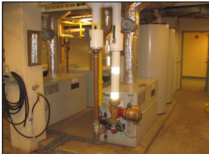
Photo No. 48: Domestic hot water boilers and storage tanks
