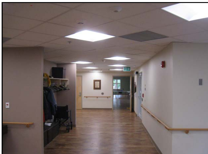
Photo No. 60: Auditorium corridor lighting
