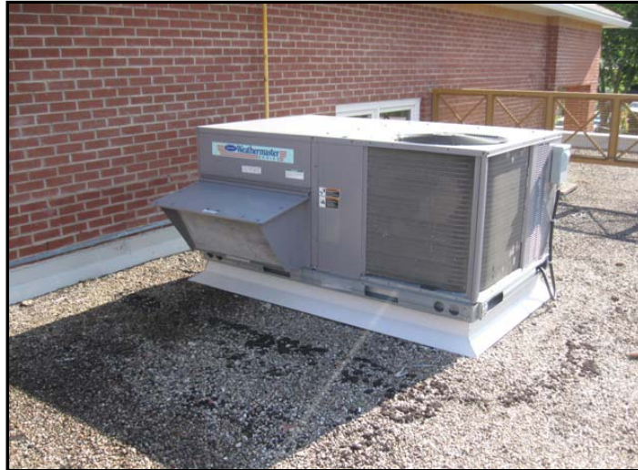
Photo No. 31: Rooftop unit
