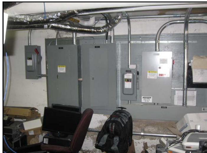
Photo No. 30: Electrical distribution panels in basement
