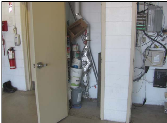
Photo No. 34: Incoming domestic water service
