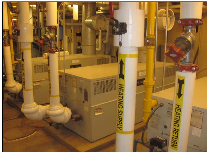
Photo No. 42: Heating boilers
