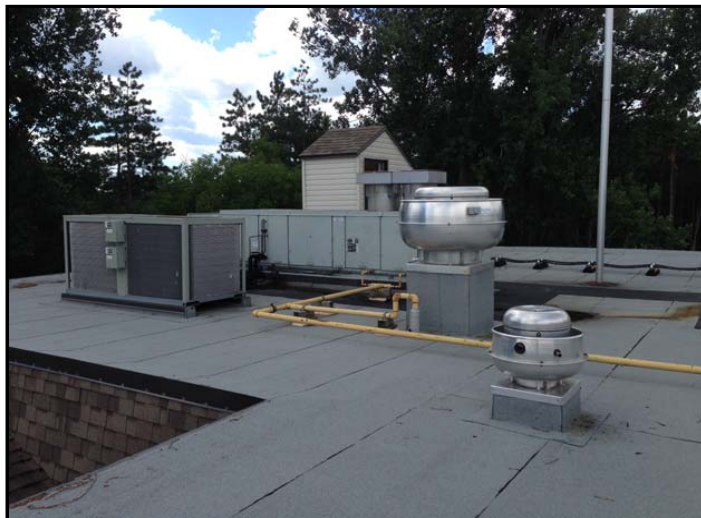
Photo No. 45: Kitchen MAU and EF
