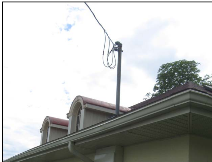
Photo No. 16: Overhead electrical service to garage
