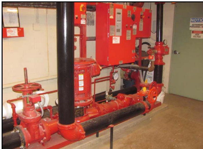
Photo No. 23: Fire pump
