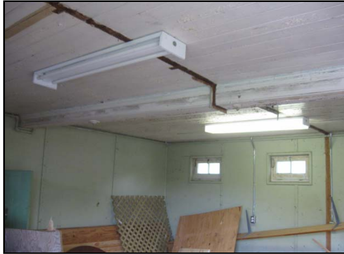
Photo No. 23: Shed ceiling-mounted lighting
