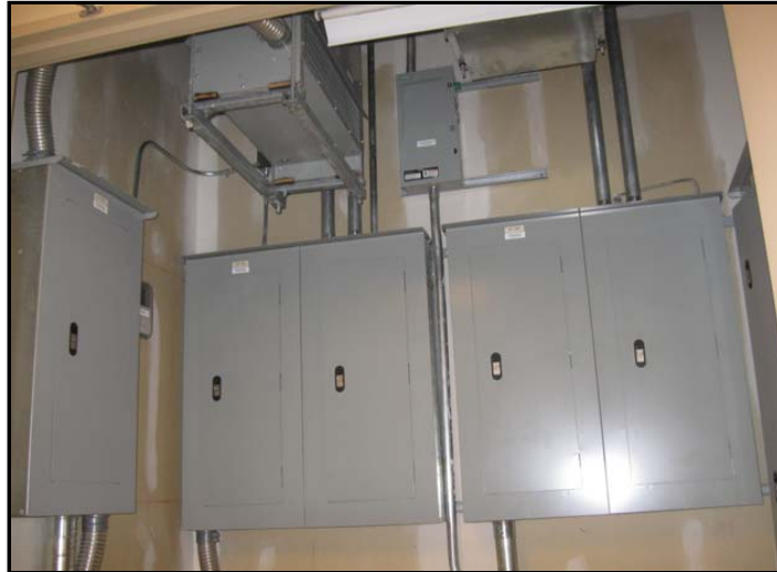
Photo No. 55: Typical normal power electrical closet
