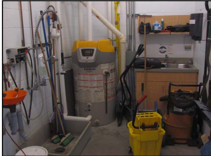
Photo No. 33: Domestic hot water tank heater
