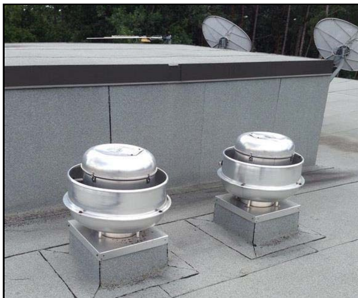
Photo No. 46: Dishwasher exhaust fans
