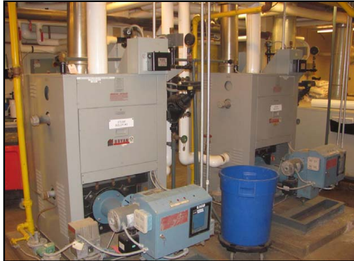
Photo No. 43: Steam boilers
