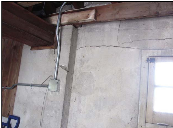
Photo No. 7: Garage cracks at east wall
