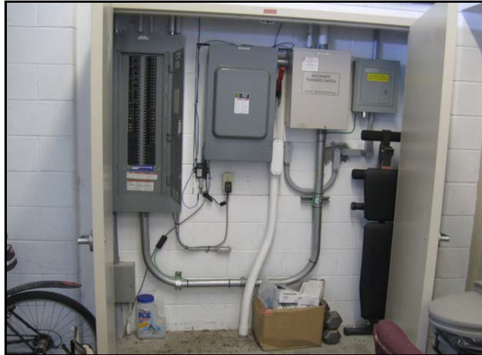
Photo No. 35: Electrical closet
