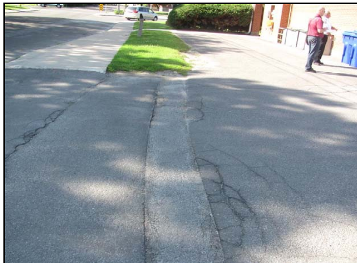
Photo No. 28: Closely-spaced cracks at Palace Rd
