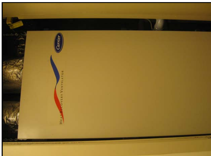
Photo No. 30: Heat recovery ventilator
