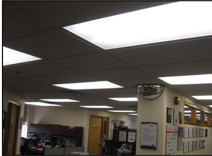
Photo No. 61: Paramedic office space lighting
