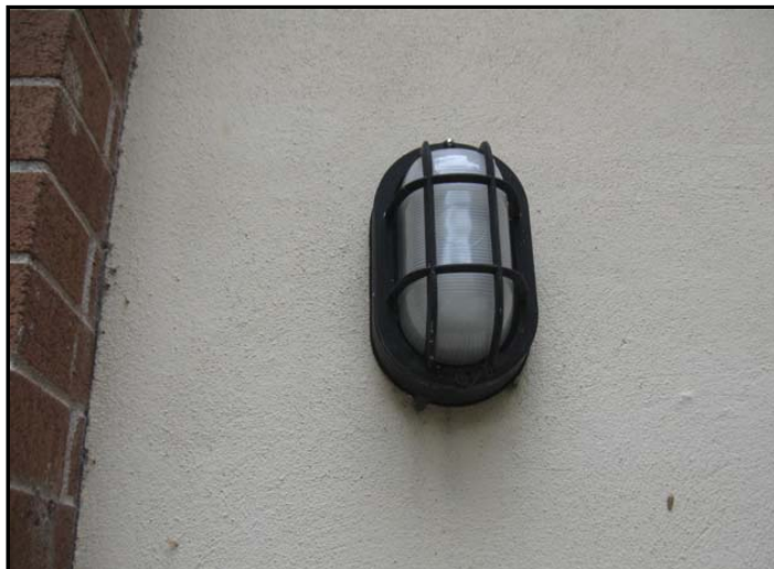
Photo No. 63: Exterior wall-mounted light
