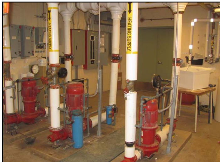
Photo No. 44: Heating distribution pumps
