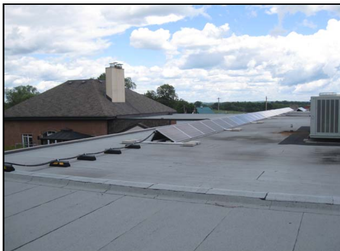
Photo No. 52: Solar panels
