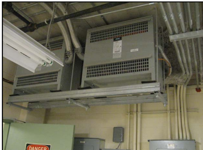
Photo No. 54: Normal power suspended transformers
