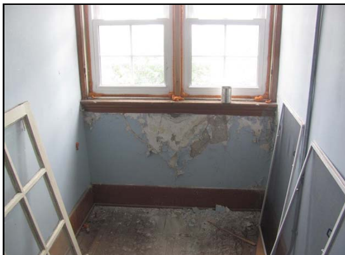
Photo No. 12: Previously leaking attic window
