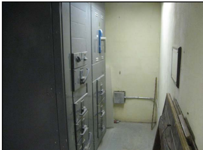
Photo No. 56: Old Switchgear serving Paramedics and Old House
