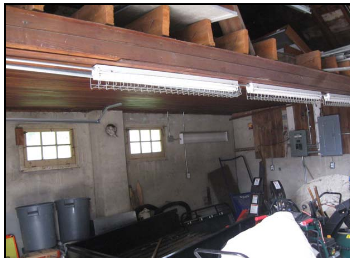
Photo No. 22: Garage interior ceiling-mounted lighting
