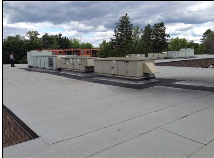
Photo No. 47: Typical RTU - Patient Care
