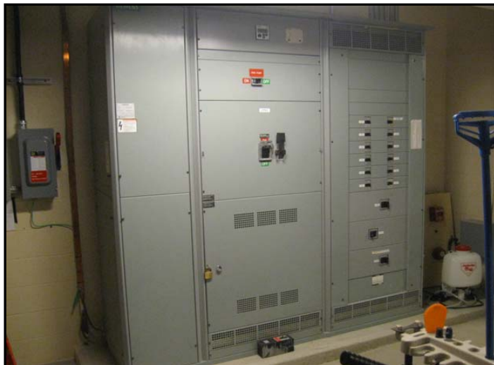
Photo No. 51: Main switchgear unit
