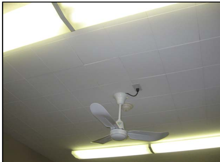
Photo No. 32: Office space lighting
