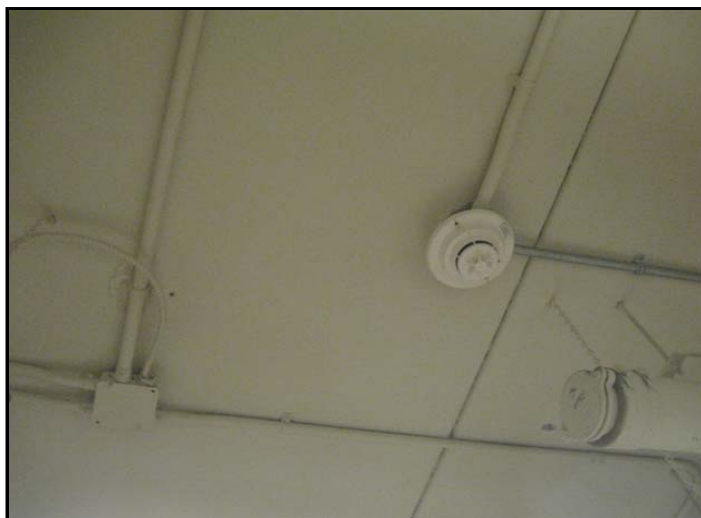
Photo No. 20: Typical heat detector
