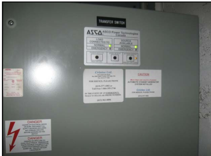
Photo No. 22: Automatic transfer switch
