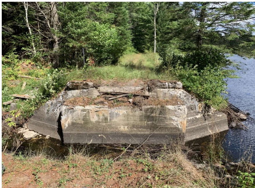
Figure 5 – Typical Deterioration of concrete on abutment and ballast walls (north shown)
