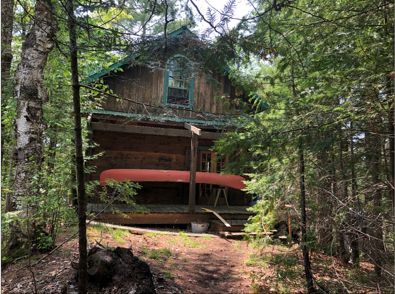
Figure 3: The end of the dwelling where the addition is proposed to be located. There is limited existing vegetation where the addition is proposed to be located.
