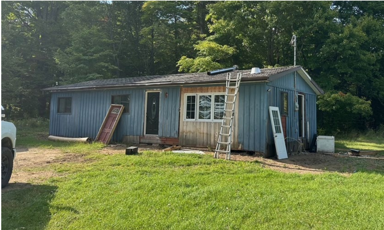
Figure 1. Image of the front of the dwelling where the deck and porch are proposed.
