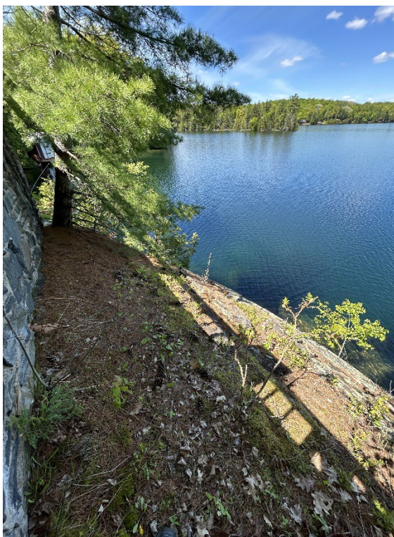
Photo 4 Exposed Bedrock Along Slope Face, North Side of Existing Dwelling, Facing West. May 2025.
