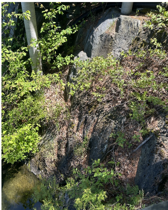
Photo 5 Slope Face and Toe, West Side of Existing Dwelling, Facing East. May 2025.
