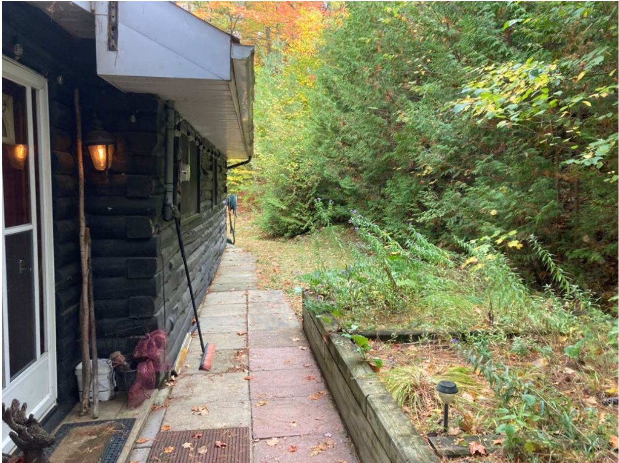
Figure 2. Area behind dwelling and assumed septic bed. The septic tanks are located in the garden bed at the foreground of the image. To the right of the garden bed is a significant slope.
