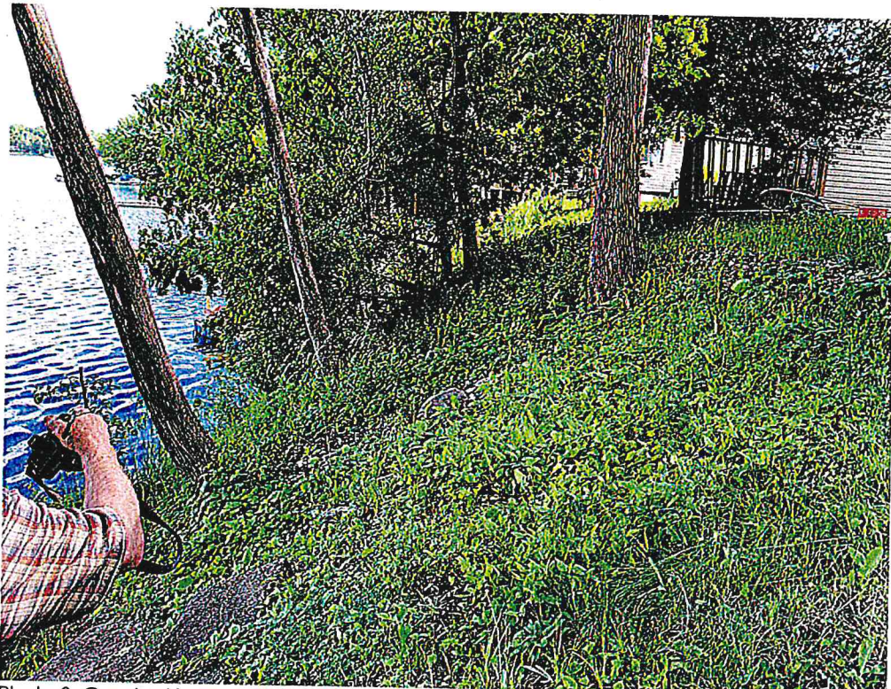
Photo 3 Gunstocking and inclination of trees on lower slope reflect creep of filled ground.
