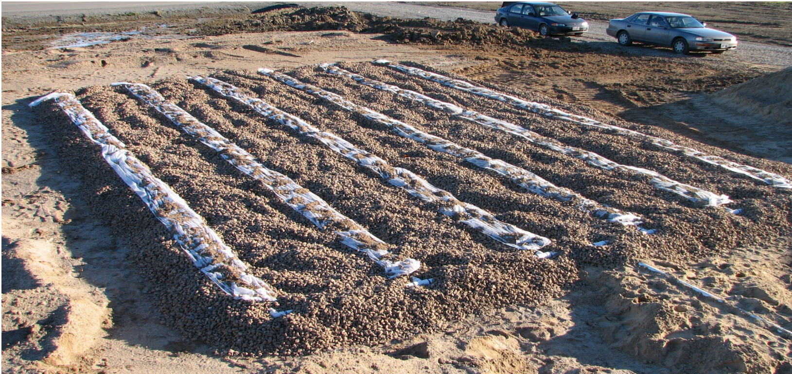
Typical Raised leaching bed
